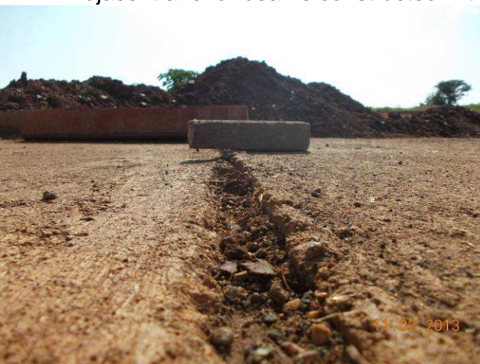
Figure 8: UTRCP Step at joint.
