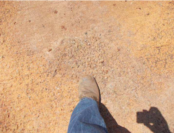
Figure 7: Inconsistent final finish.
