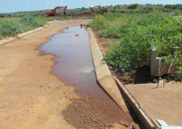
Figure 6: Ponding on UTRCP.
