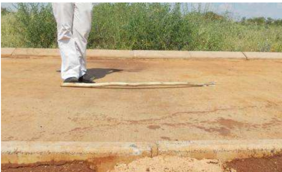
Figure 3: Sagging UTRCP due to sagged layerworks.
