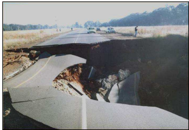
Plate 14. Sinkhole on Venterspost-Westonaria Road, West Rand (1960's) as a result of dewatering (Photo from Oberholzer Ground Stability Group).
