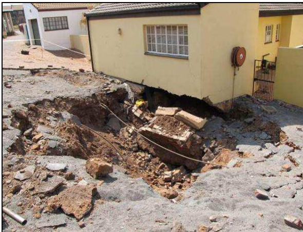
Plate 11: Sinkhole in Valhalla, Tshwane (2008), Due to a leaking service. (Photo by S Richardson).
