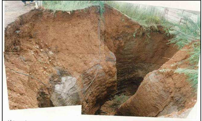
Plate 6: Sinkhole on Waterkloof Airforce Base, Tshwane (1996), due to poor surface drainage. (Photo from CGS archives).
