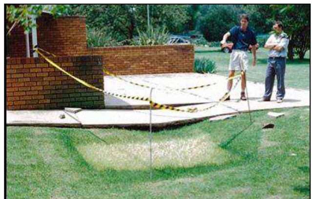
Plate 20: Subsidence at Irene Research Institute, Tshwane (1990's), due to a leaking service (Photo from CGS archives).
