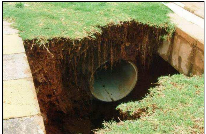
Plate 4: Sinkhole on Cantonments Road, Lyttelton, Tshwane (1995), due to a leaking service (Photo from CGS archives).
