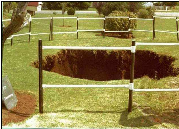
Plate 3: Sinkhole in Finus Road, Valhalla, Tshwane (1973) due to a leaking service (Photo from CGS archives).
