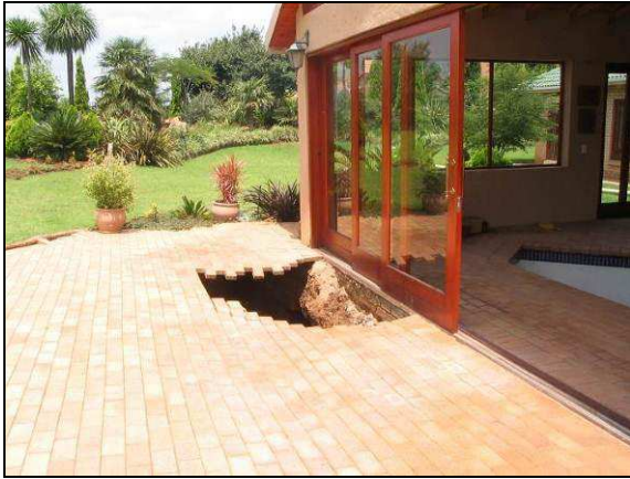
Plate 9: Sinkhole at house in Cornwall Hill (2006). Due to a leaking swimming pool (Photo by A.C. Oosthuizen, CGS).
