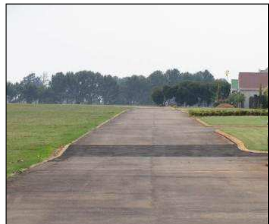
Plate 26. Dewatering subsidence, Elandsfontein, Ekurhuleni (2009), due to dewatering (Photo by G.J. Heath, CGS).
