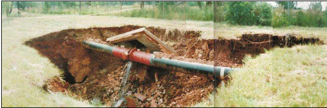
Plate 2. Leaking pipeline in Alaric Road, Valhalla (1996). (Photo from CGS archives, referenced by Waltham et al. , 2005 as taken by/from F. Bell).
