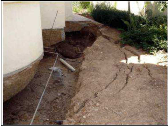
Plate 23. Subsidence in Irene, Tshwane (2010), due to a leaking service (Photo from CGS archives).
