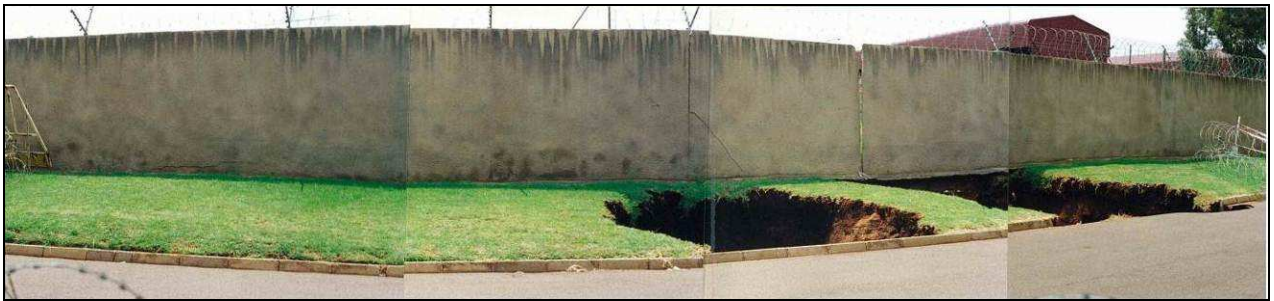
Plate 7: Sinkholes outside boundary wall of Waterkloof Airforce Base, Tshwane (1996), due to poor surface drainage (stormwater damming up behind wall). (Photo from CGS archives).
