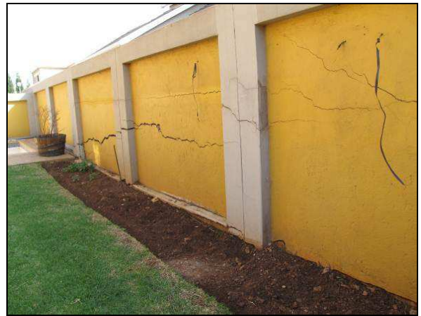
Plate 22. Subsidence in Irene, Tshwane (2009), due to a leaking service (Photo by A. C. Oosthuizen, CGS)
