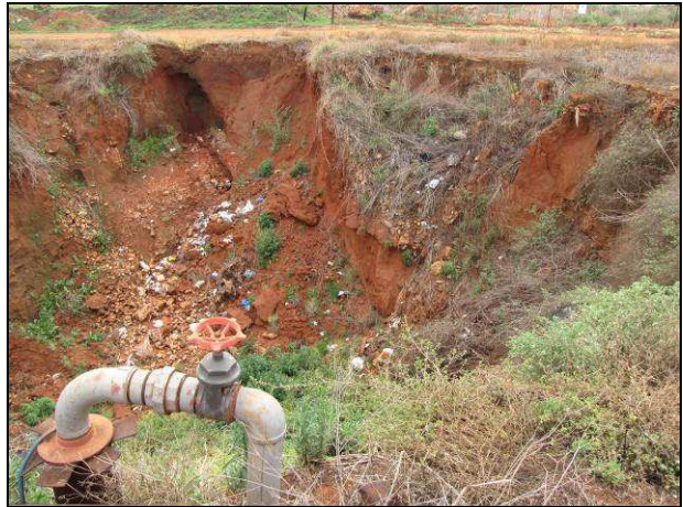
Plate 16. Sinkhole in Elandsfontein, Ekurhuleni (2007) as a result of dewatering (Photo by G.J Heath, CGS)
