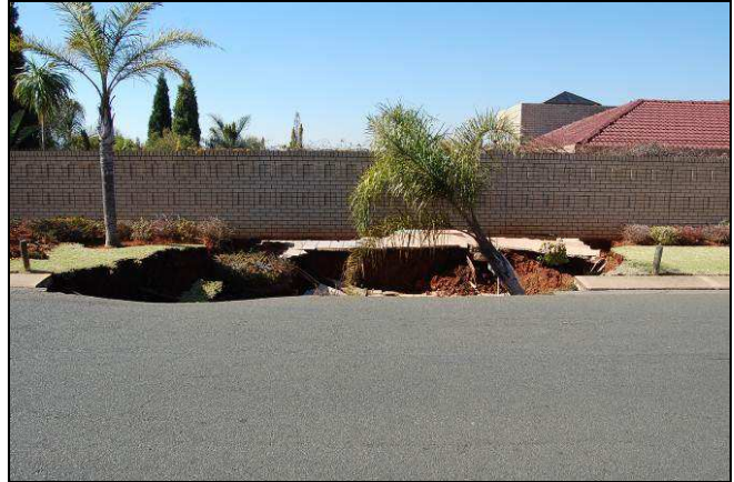
Plate 10: Sinkhole In Laudium (2007), due to a leaking service. (Photo by A.C. Oosthuizen, CGS).
