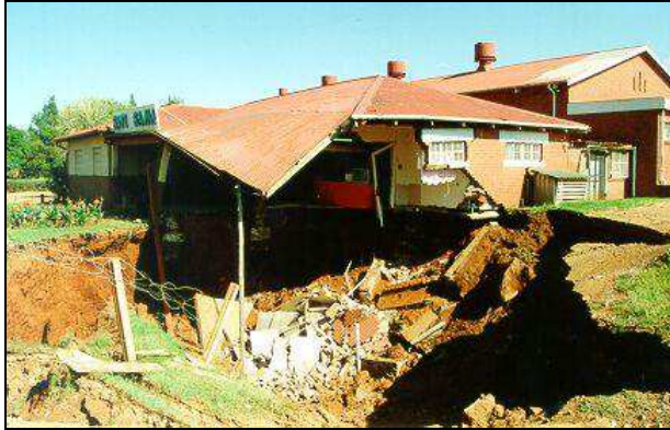
Plate 5. A house in Centurion (military area) destroyed by a sinkhole (1995). (Photo from CGS archives, referenced by Waltham et al., 2005 as by/from F. Bell).
