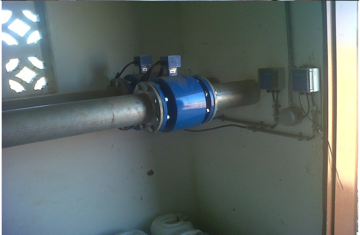
Water pumps and water meters in a pump house of sugar cane farm
