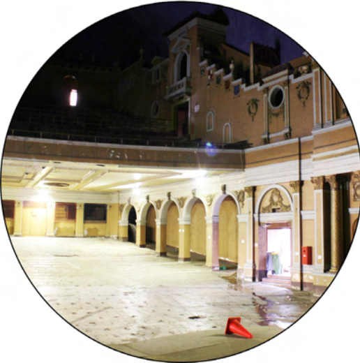
Fig. 3.19.2 Current building failures: inaccessible first floor gallery due to structural failure (Author 2013)
