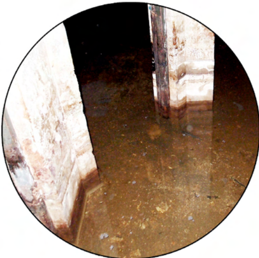
Fig. 3.19.3 Current building failures: flooded basement (Author 2013)
