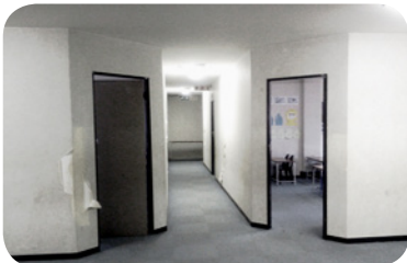
Figure 3.3(a): Corridor with unkempt walls and no natural lighting or ventilation. (Photo by: Author)
