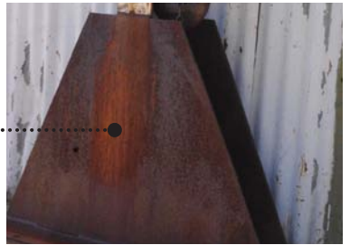
steel base plates .....
