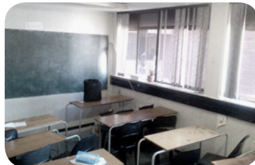
Figure 3.3(b): Tiny classrooms with inadequate sunlight and ceiling height. (Photo by: Author)
