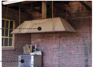
old extractor fans .....
