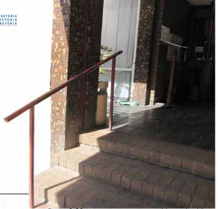
Figure 2-39 Main entrance not accessible to wheelchairs
