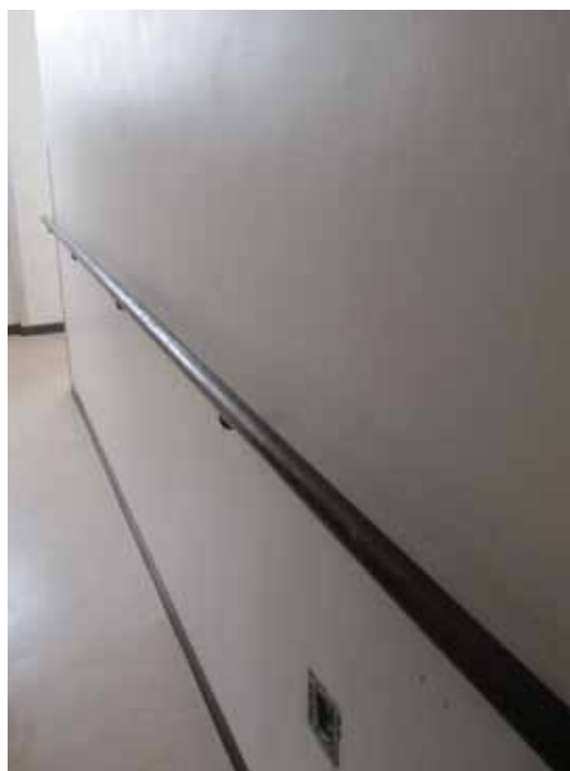
Figure 7-34 Removed handrails (Author,2013)
