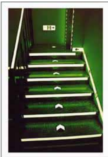
Figure 8-20 Photo-luminescence textile strips
