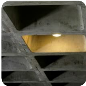
Figure 111: Zone B coffer slab lighting appropriation [Uni-span, 2013]
