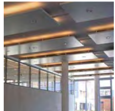
Fig. 8.62. light fittings hidden above panel
