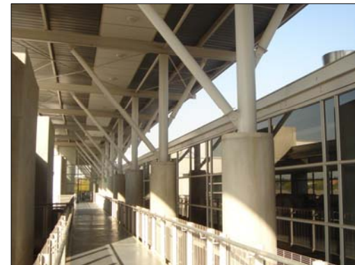
Fig 3.10 (c): Expression of Structure in the Law Faculty Building in the Circulation Spine
