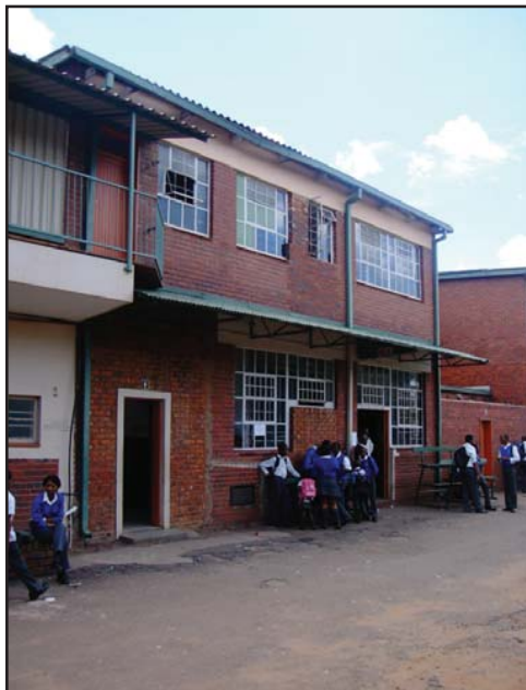
fig.4.10. Various alterations are visible on the facade of Berea Park School. The structure was originally used for warehousing purposes.
