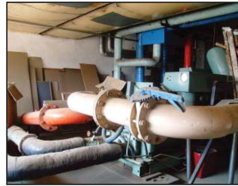
fig.5.34. Mechanical ventilation room on northern platform
