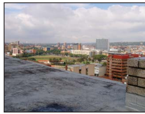
fig.5.44. Unsafe periphery with hollow brick columns ending in stubs
