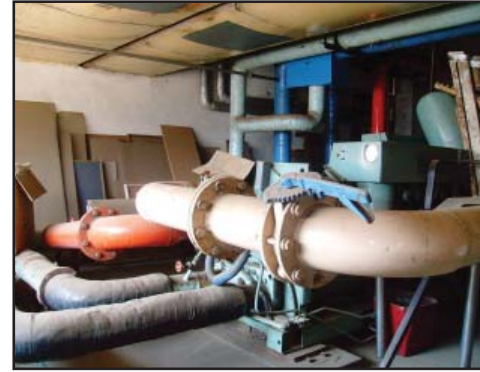
fig.5.34. Mechanical ventilation room on northern platform
