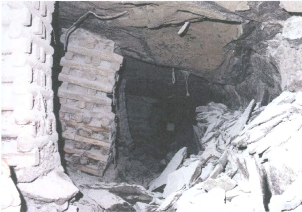
Figure 4.20 - Merensky Reef - no siding. Severe spalling down dip
