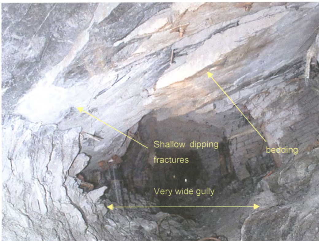
Figure 4.27 - Basal Reef – the effect of a lagging siding on hangingwall conditions – view from face area looking back along gully at 1700m
