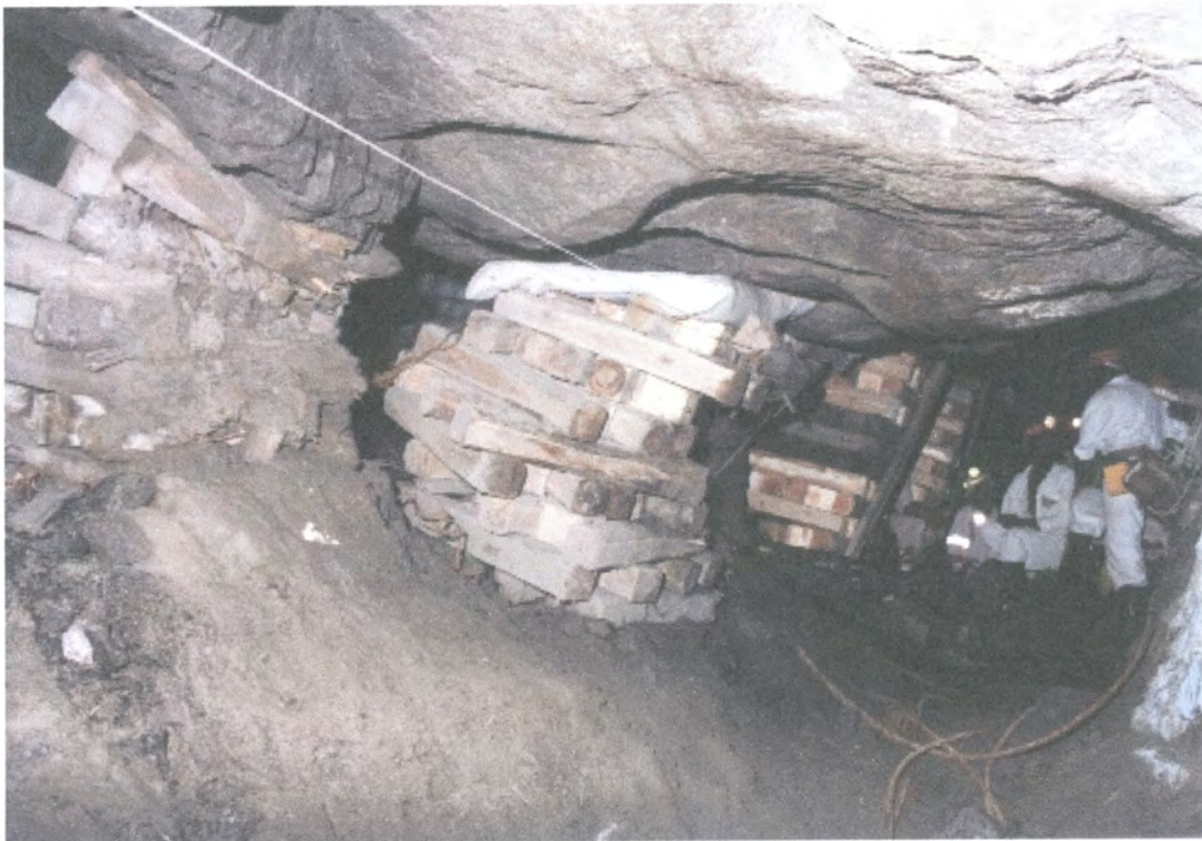
Figure 4.50 – Gully shoulder and hangingwall unevenness results in uneven compression of pack and its eventual disintegration
