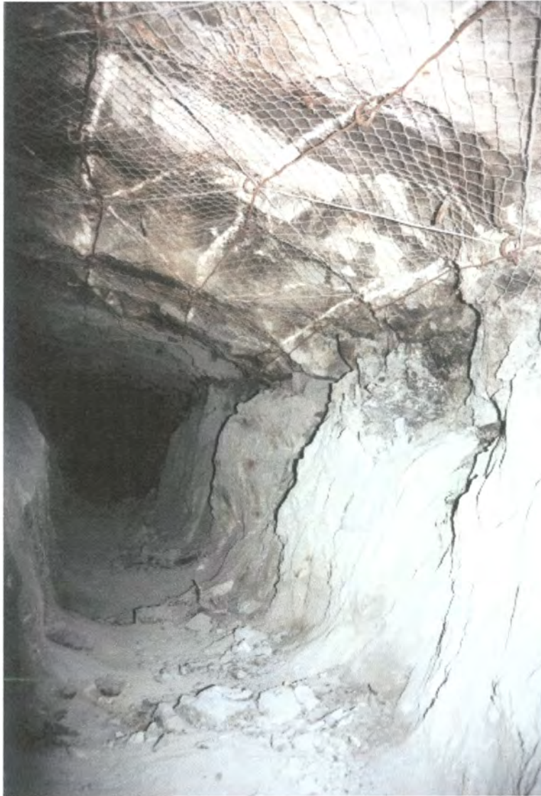
Figure 4.19 - Merensky Reef gully where a crush pillar lies on the gully edge and during crushing has damaged the hangingwall resulting in mesh and lacing application to control minor falls
