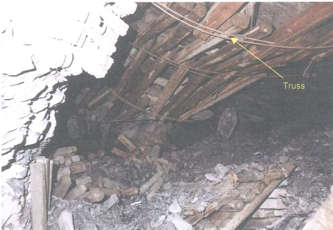
Figure 4.39 – Roadway after seismic damage – packs collapsed, trusses and hangingwall intact (after rockburst)
