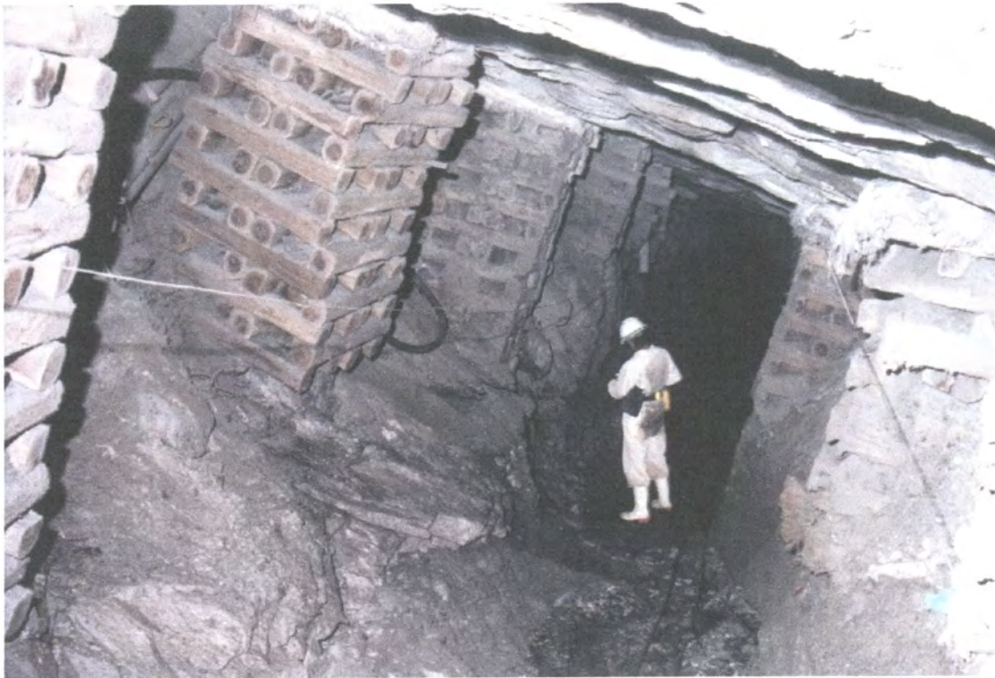
Figure 4.22 – Merensky Reef - footwall lifted gully in wide heading. Due to down dip sidewall integrity, all packs are normal to dip
