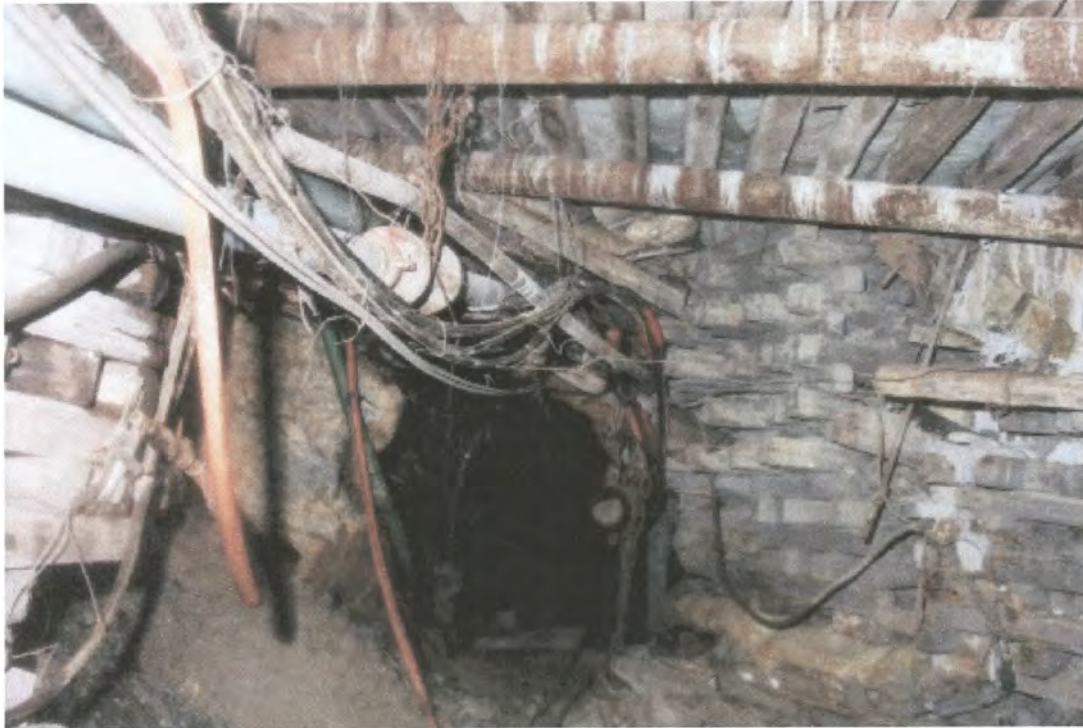
Figure 4.42 – Strike gully on the Carbon Leader reef at 2900 m depth, where a stable long term access has been achieved through using sets and void filling
