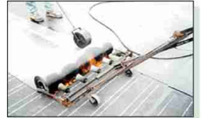
Figure 6.09 Example of roof treatment: Application of a modified bitumen cap sheet, torched on
