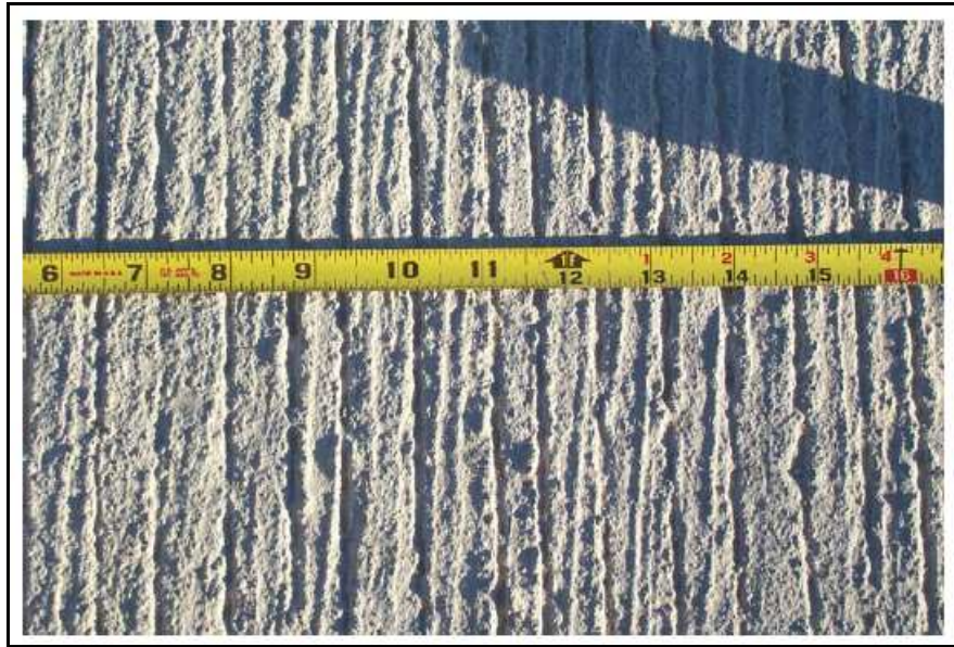
Figure 2: Longitudinally tined concrete, direction of travel from bottom to top (Karamihas and Gillespie, 2002).
