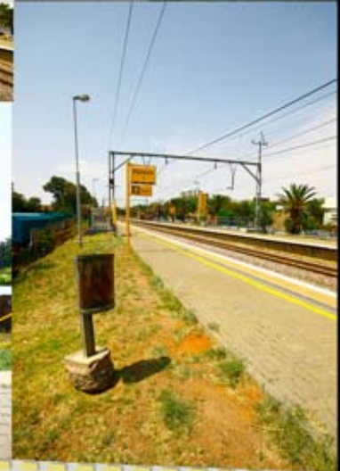
fig. 3.40_ Platform embankment, vandalized litter bin
