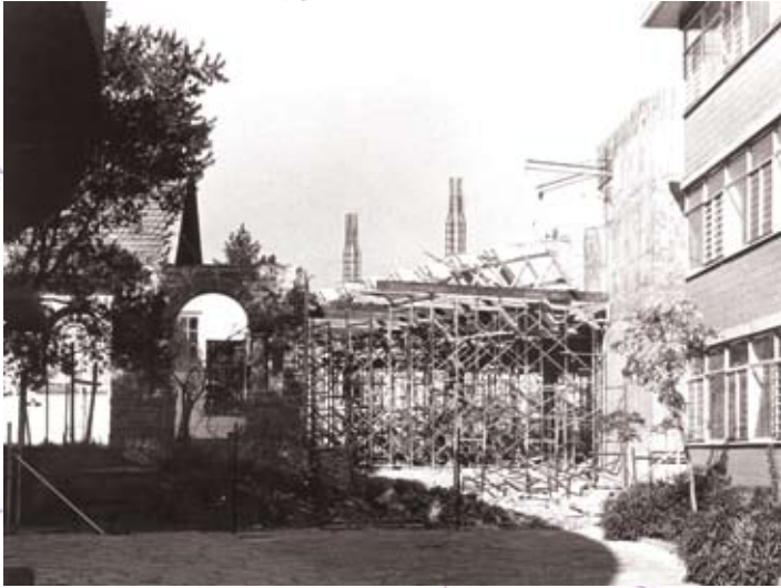
Figure 3.3: Construction of the New Merensky Library, to the left the partial demolition of the Old Chemistry (the arches were left in tact)
