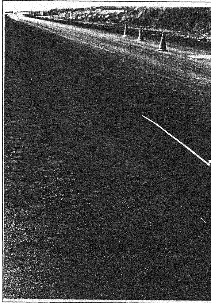
Figure 9.7 General View of Kriel Colliery Site 1, showing rutting and damage to wearing course.
