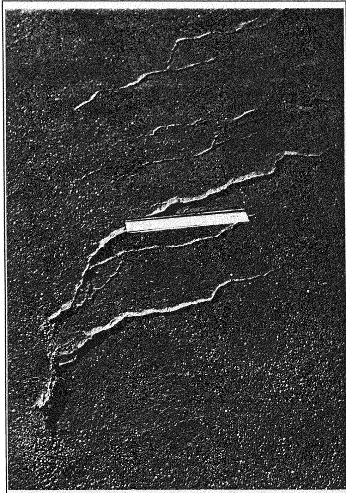
Figure 9.20 Cracking and pushing out of wearing course in centre of road, Kromdraai Colliery Site 1.
