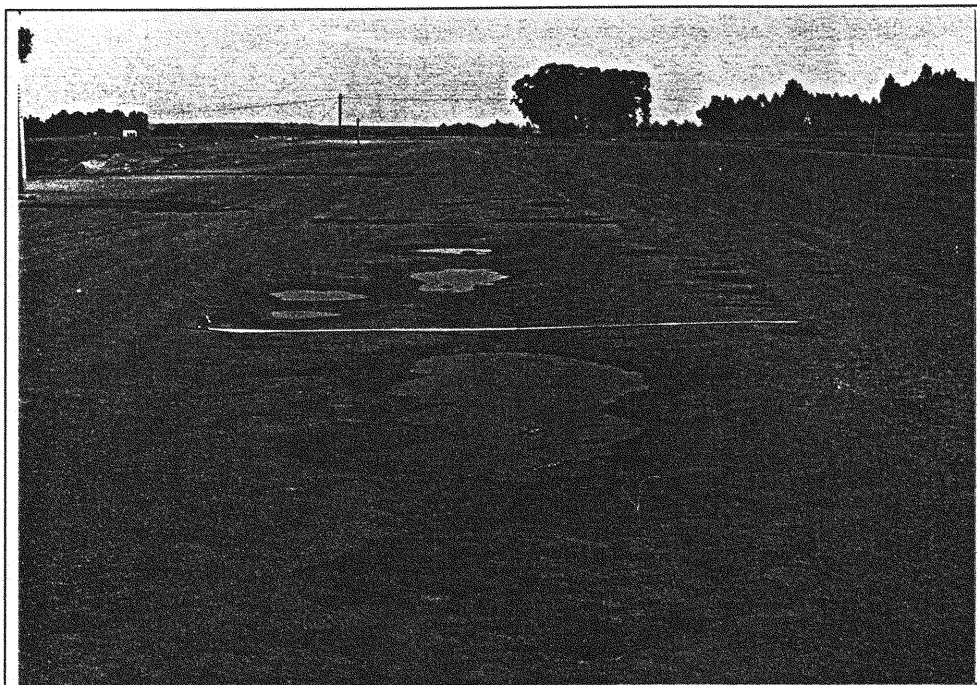
Figure 9.28 Potholing as a result of localised soft spot in newly constructed and trafficked site 3 road at SACE Kromdraai Colliery.
