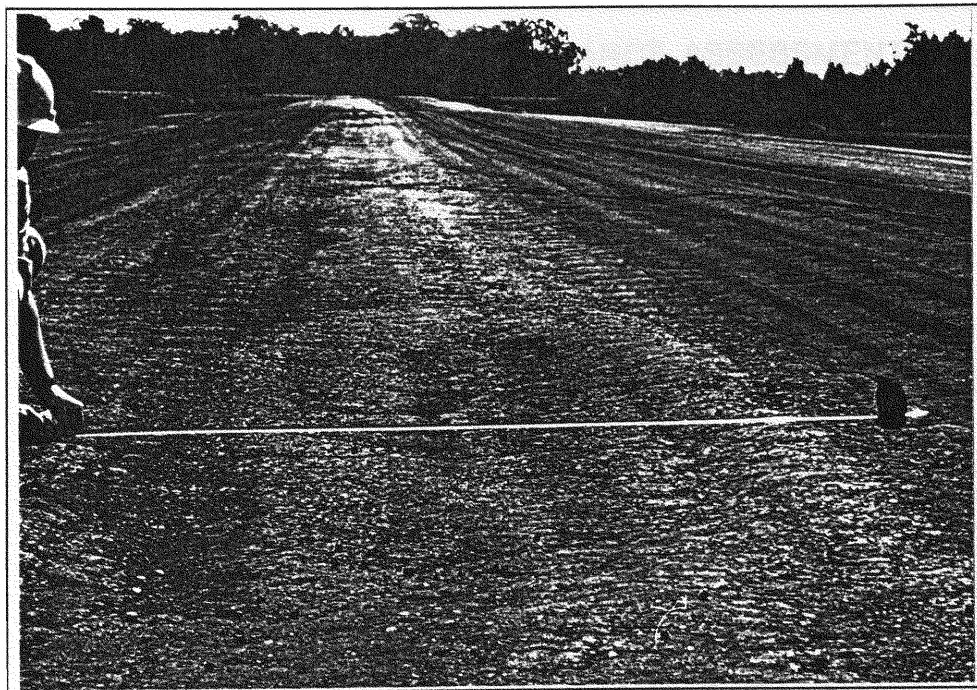
Figure 9.41 Slip cracks and deformation of sub-base, New Vaal Site 2.
