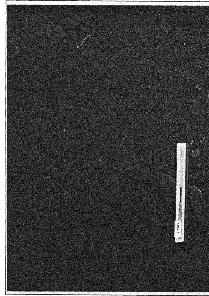
Figure 9.8 Crocodile cracking and large stones in wearing course, Kriel Colliery site 1.
