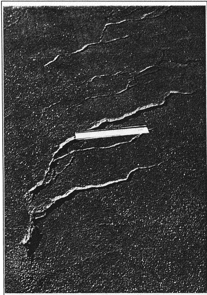
Figure 9.20 Cracking and pushing out of wearing course in centre of road, Kromdraai Colliery Site 1.
