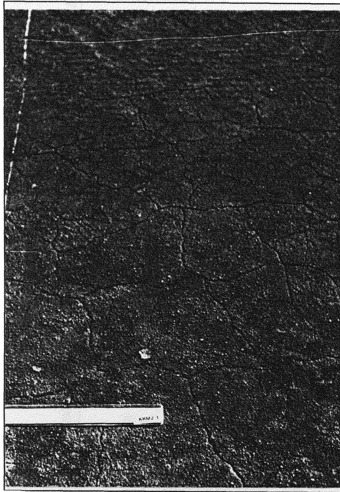
Figure 9.24 Typical crocodile cracking defect at SACE Kromdraai Colliery site 2.
