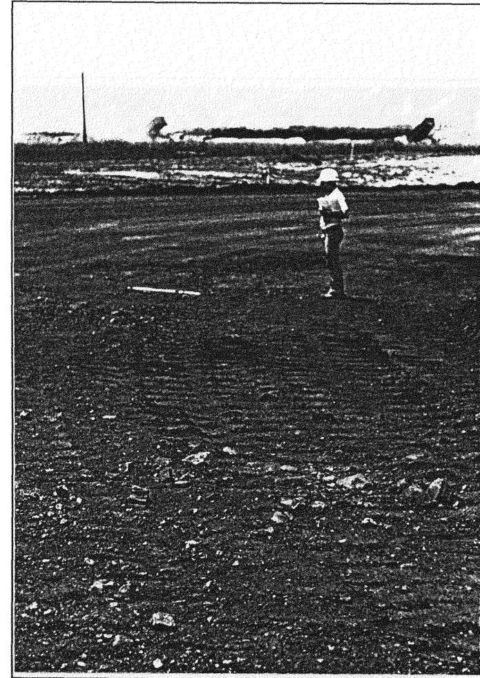
Figure 9.40 Typical damage to wearing course on bends, showing exposed stones, New Vaal Colliery Site 2.
