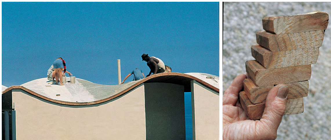
Figure 7.34. Left: The roof of Die Es under construction c.1965 (Fagan, 2012b). Right: Layered construction of Die Es roof (Fagan, 2012b).
