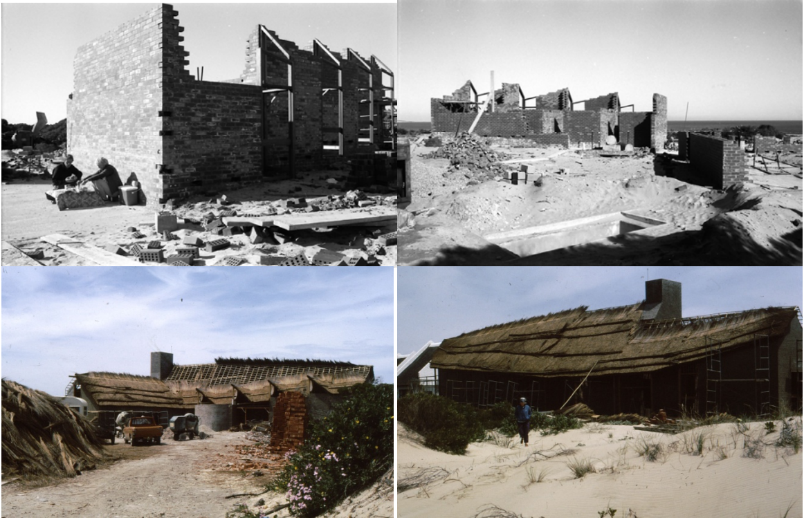
Figure 8.35. Top left: The Fagans picnicking alongside the partly constructed building. Top right: Walls constructed to roof height. Bottom left: Roof under construction viewed from site entry point. Bottom right: Roof under construction as viewed from sea edge (All Fagan archive job no. 8011, slide collection IC).
