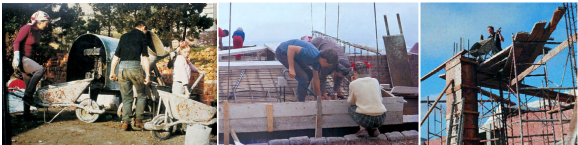
Figure 7.37. Fagan and family at work on Die Es (1965). On the left Fagan can be seen with Gwen hauling concrete with their wheel barrows while his son Hennie fixes steel for the first floor in the centre picture. On the right Fagan pours concrete into the formwork of one of the columns, a job he notes (2012b) that no one else was prepared to do from the rickety scaffolding!
