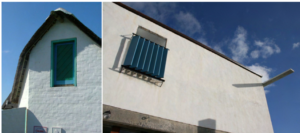
Figure 7.9. Left: Bagged and painted brickwork to House Swanepoel in Cape St. Francis (1980) (Author, 2005). Right: Honest expression of different materials at Die Es (1965) (Author, 2008).
