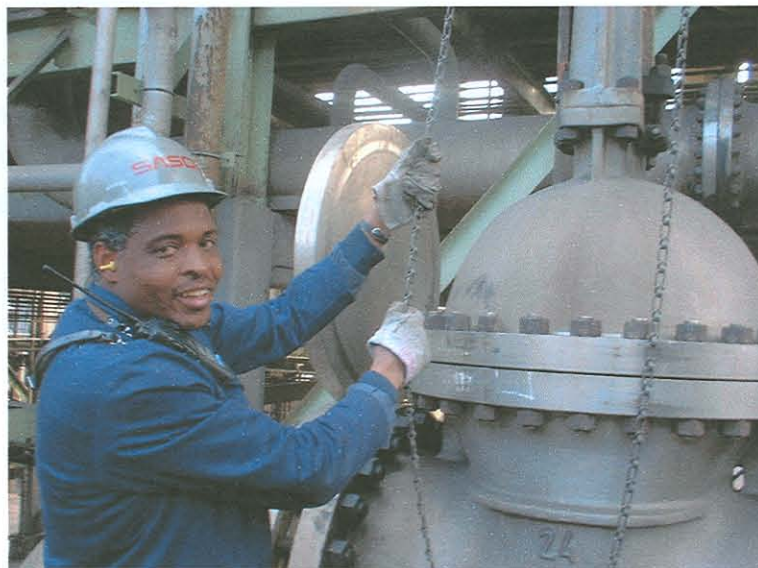
Figure 4.6: 24" Wedge gate valve being closed
