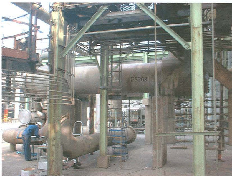
Figure 4.1 ES 208 Tail gas shell-and-tube heat exchanger
