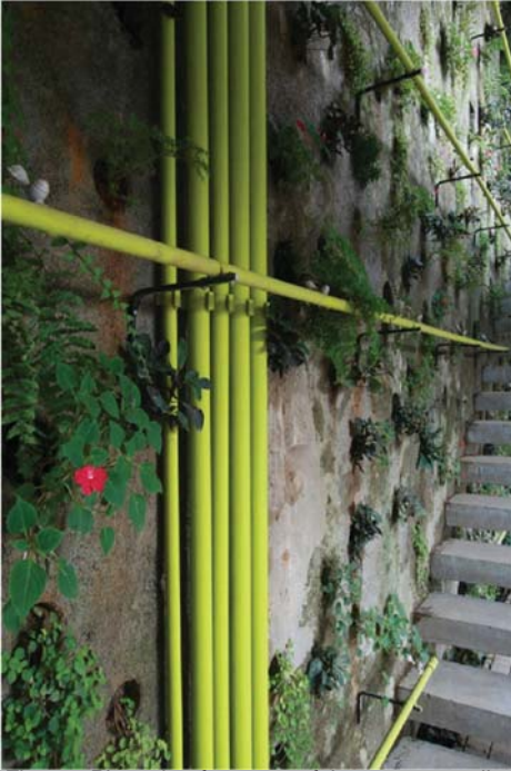
Fig.288:Pipes that form part of the water recycling system in Harmonia 57 [Source: http://www.architonic.com/aisht/harmonia-57-triptyque-architecture/5100477 ]
