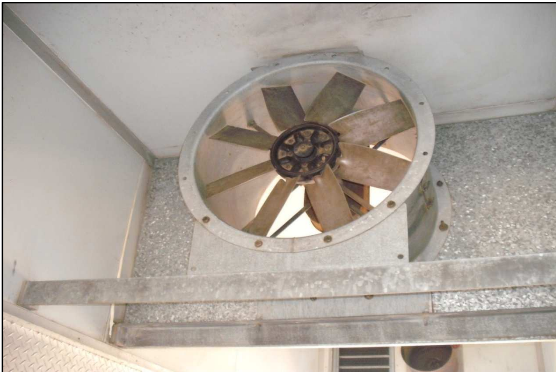
Figure 4-16 Main fan on support beams (Viewed from down-stream side)
