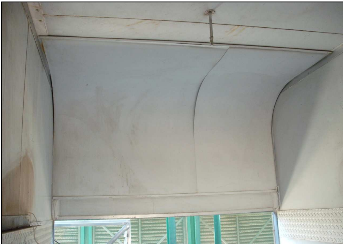
Figure 4-26 Turning vane (Viewed from downstream fan position)
