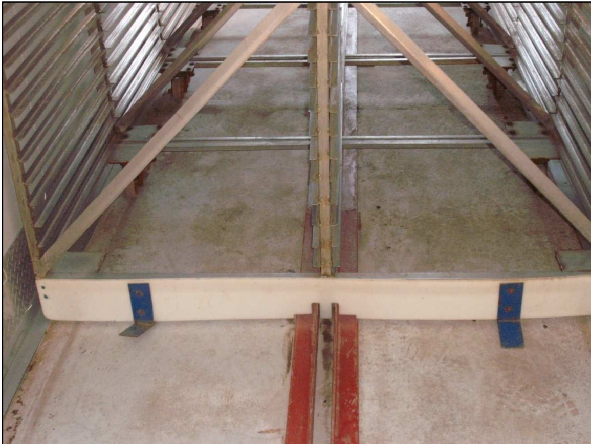
Figure 6-5 Blanking off plate placed before first trolley
