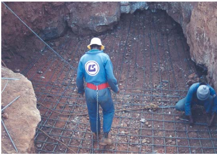
Plate 2: Rehabilitation of an old sinkhole, placement of steel mesh (courtesy J Van Der Merwe)
