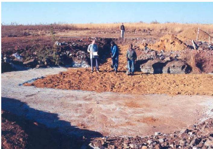
Plate 3: Rehabilitation of an old sinkhole, infill of fine material and placement of concrete layer (courtesy J Van Der Merwe)
