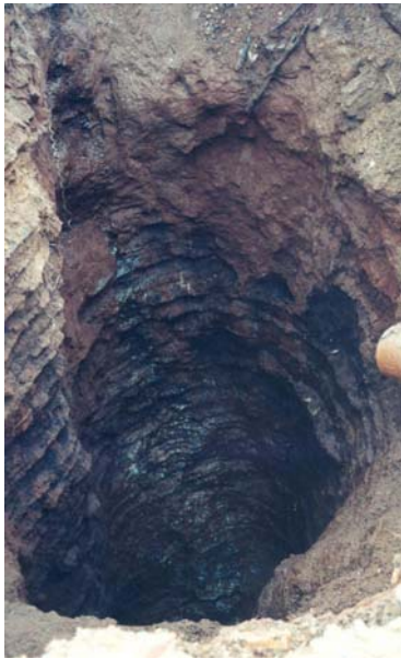
Plates 4 and 5: Sinkhole through fill material (courtesy J Van Der Merwe)
