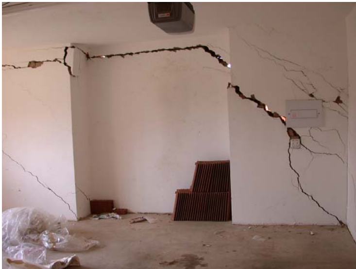
Plate 6: Cracking of structure due to subsidence
