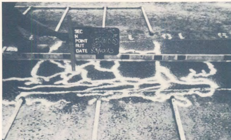
(c) Maximum rut of 80 mm on MDD12. Note the fatigue cracking of the asphalt layer. E80s on wet test section: 6,8 \times 10^6
