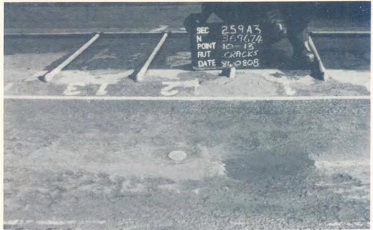
(b) Pumping on Section 2 through MDD hole at measuring point 12 and longitudinal cracks.
