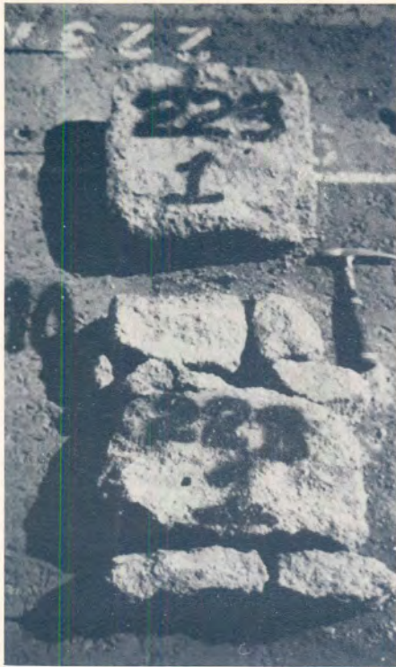
(a) Recovered upper subbase after 20,6 ME80s on SECTION 1 (saturated). Layer cracked and fractured (Measuring points 11 to 12).
