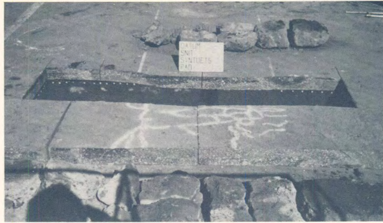
(a) Cross profile across the test Section 1. Note the heaving of the asphalt as a result of the erosion action inside the trafficked area during the EPWP state.
