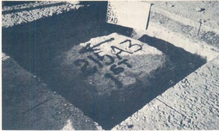
(a) Successful recovery of a solid block of stabilized material from the upper stabilized subbase layer.
