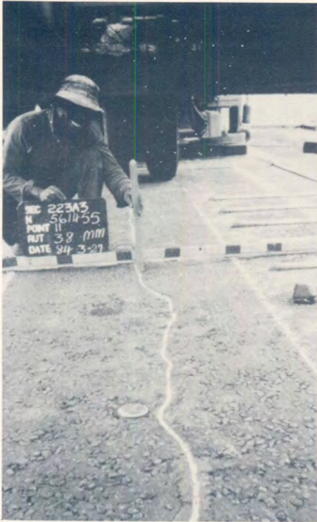
(a) Maximum permanent deformation of 38 mm at the crack after water introduction.
