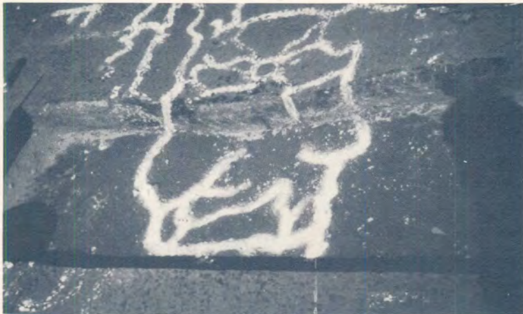
(b) Visible cracks on top of the upper stabilized subbase layer after the removal of the asphalt in (a).
