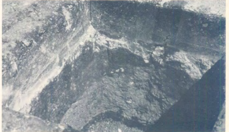
(b) Relative low pH zone at the position of the crack (dark red colour – high pH zone), determined with Phenolphthalein.
