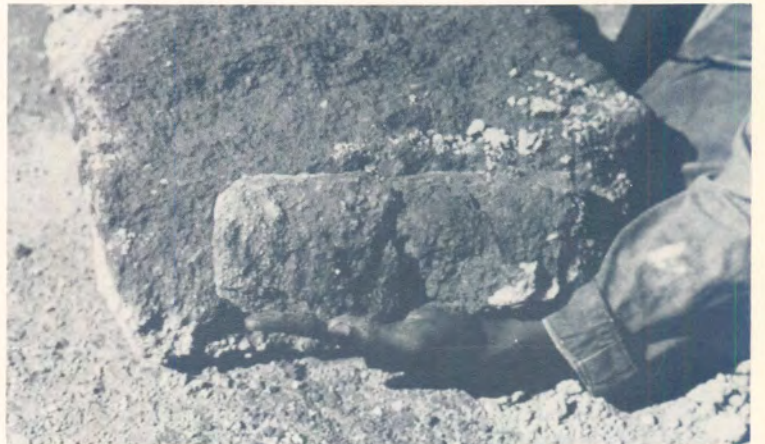
(c) Note the discolouring on the side of the block next to the crack.
