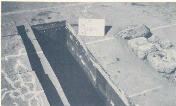
(c) Phenolphthalein indication of continuous relative high pH within both the upper and lower stabilized subbase layers.
