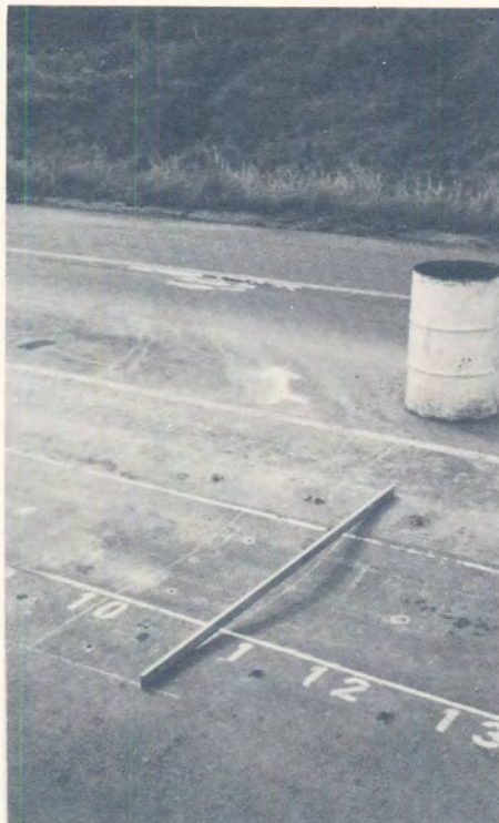
(b) Real road failure next to Section 2 in the normal trafficked lane during the time of HVS testing on Section 2.
