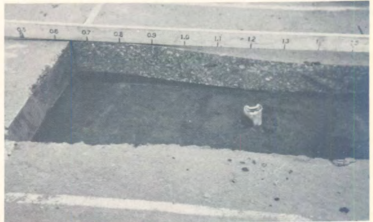
(b) Sideways (horizontal) pumping (erosion) of the lime treated Berea Red upper subbase at the bottom of the heaved asphalt on Section 1.
