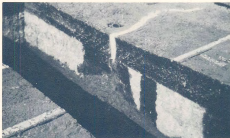
(b) Relative low pH zone at the position of the crack and the bottom of the lower subbase layer. This zone was carbonated, determined with HCL solution. The dark red area is the relative high pH zone.
