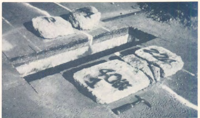
(d) Recovered upper and lower subbase layers from SECTION 2, measuring points 3 to 4, after 280 494 E80s. Note, only non-traffic associated cracks in the blocks.
