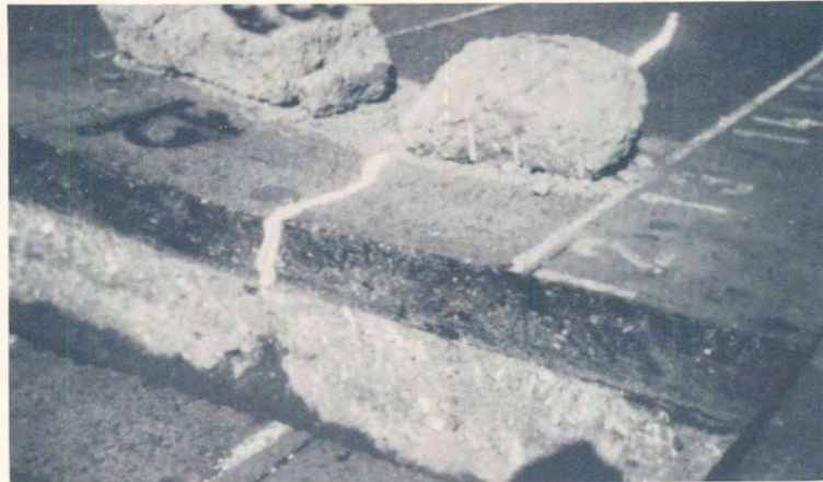
(a) Moisture regime at the crack at measuring point 12 on SECTION 1.
