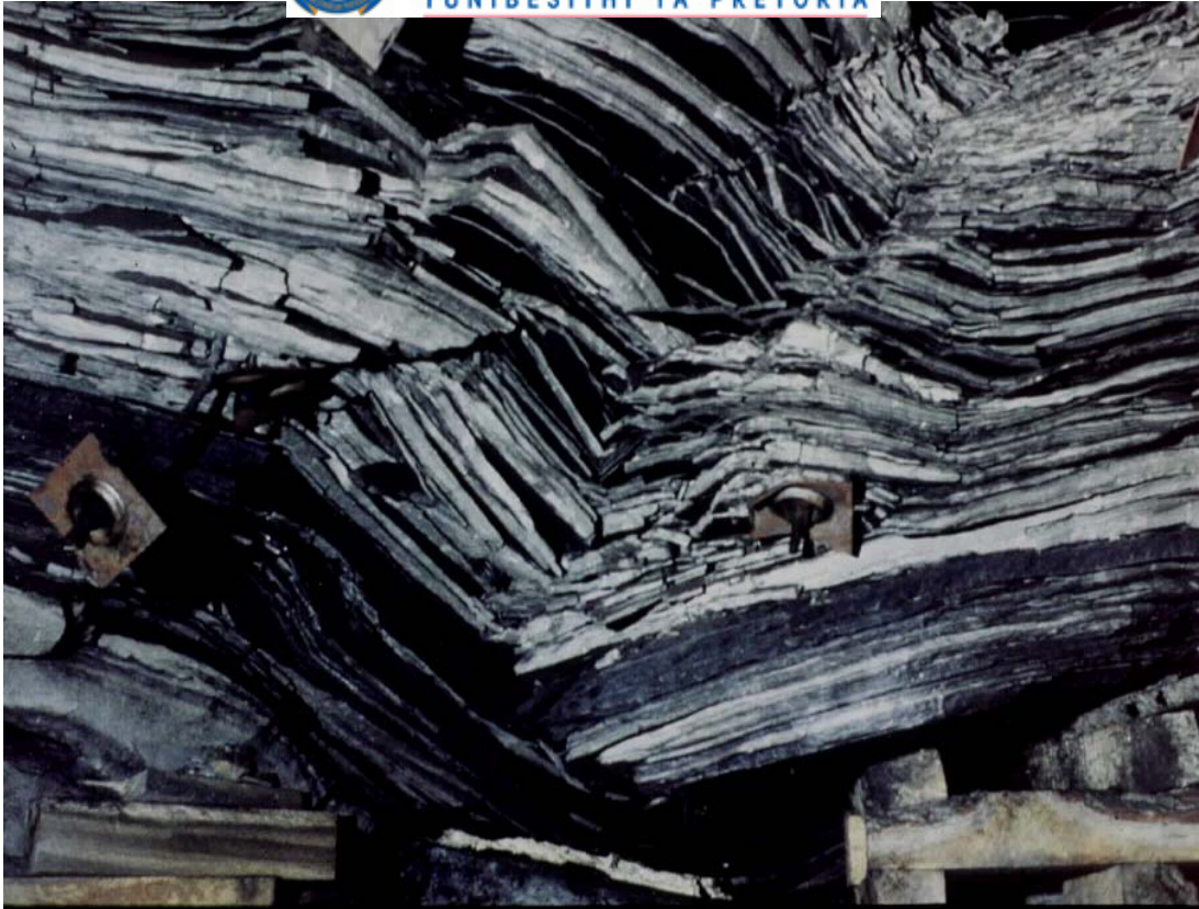
Figure 7-4 An example of roof-softening in a coal mine in the USA (courtesy of Dr. C. Mark)
