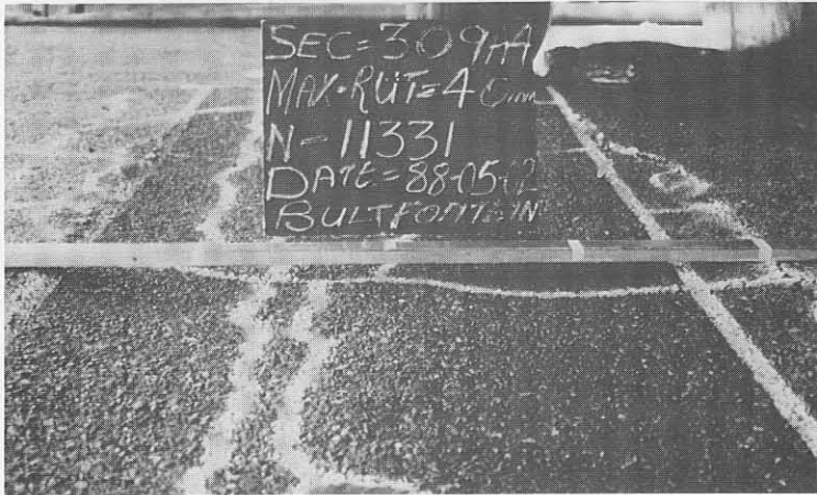
(a) Fatigue cracking and deformation (maximum 40 mm) after 11 331 repetitions.
