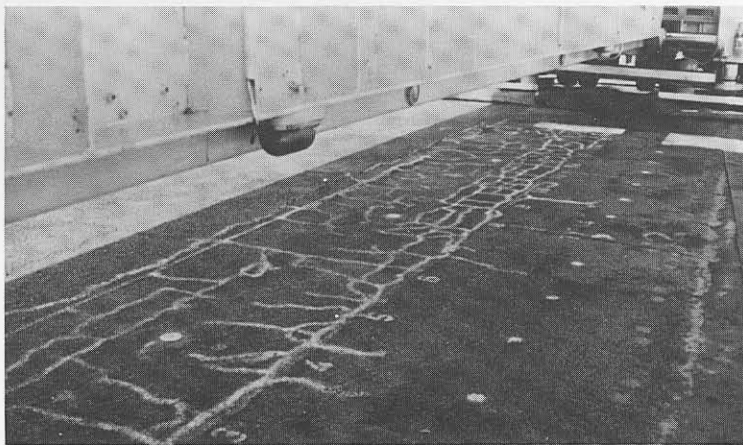
(c) Fatigue cracking after approximately 2,45 \times 10^6 70 kN repetitions.
