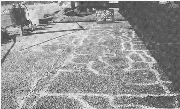
(b) Fatigue cracking after approximately 1,46 \times 10^6 70 kN repetitions.
