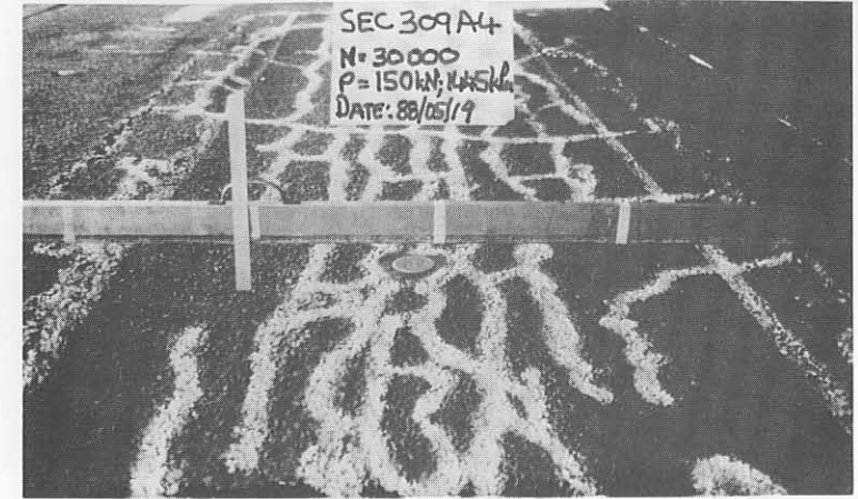
(b) Further fatigue cracking and deformation (maximum 64 mm) after 30 000 repetitions.
