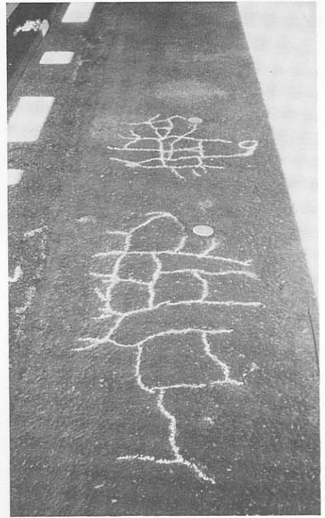
(b) Fatigue cracking (100 mm × 100 mm blocks) after approximately 1,0 \times 10^6 repetitions (E80s).
