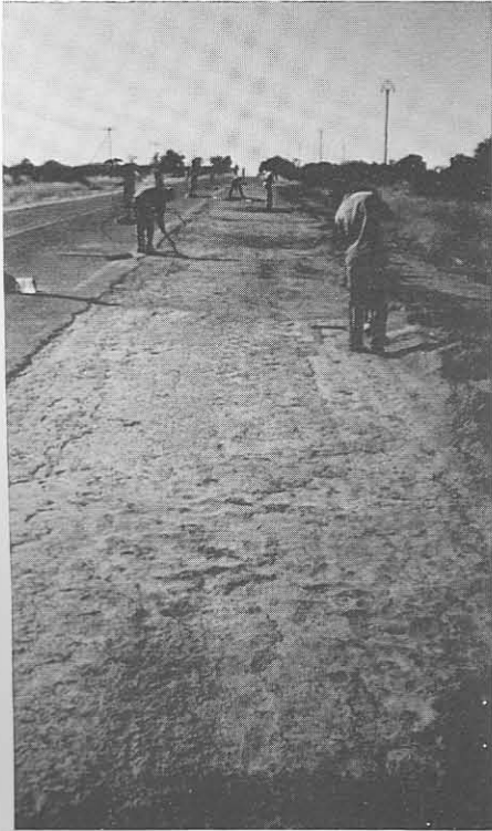
(a) Brooming of surface of the cemented base layer after the "crack and seat" operation, before the application of the prime coat.
