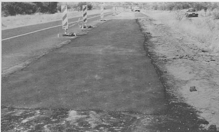
(c) Final surface of the 35 mm asphalt premix section (40 m in length).
