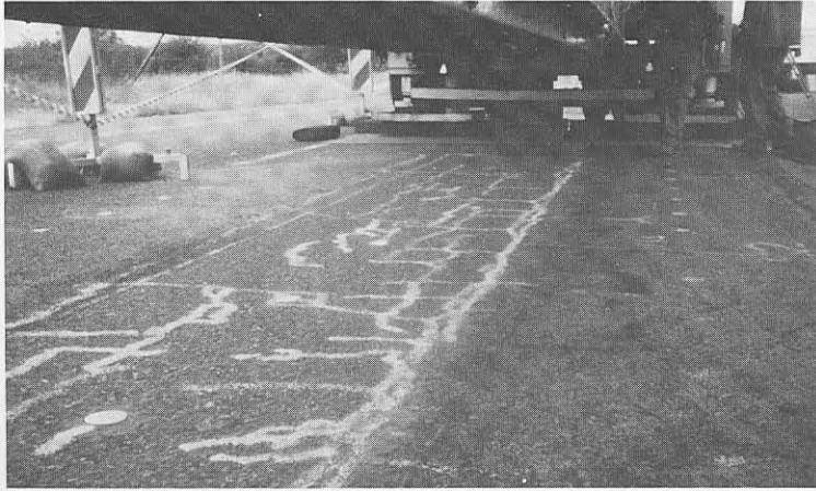
(a) Fatigue cracking after approximately 731 783 70 kN repetitions.
