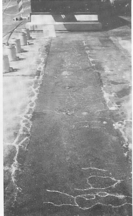
(c) Final cracking and deformation (approximately 22 mm) on section.
