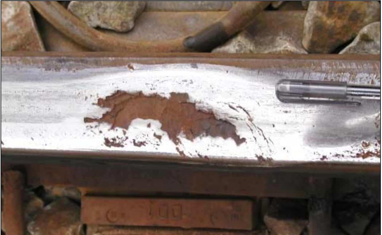
Figure 4-1: Skid mark on rail running surface
