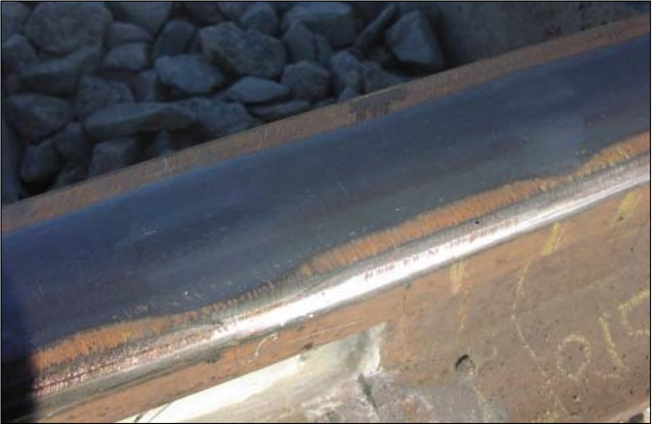
Figure 4-5: Dip joint identified by two wider patches on the contact band
