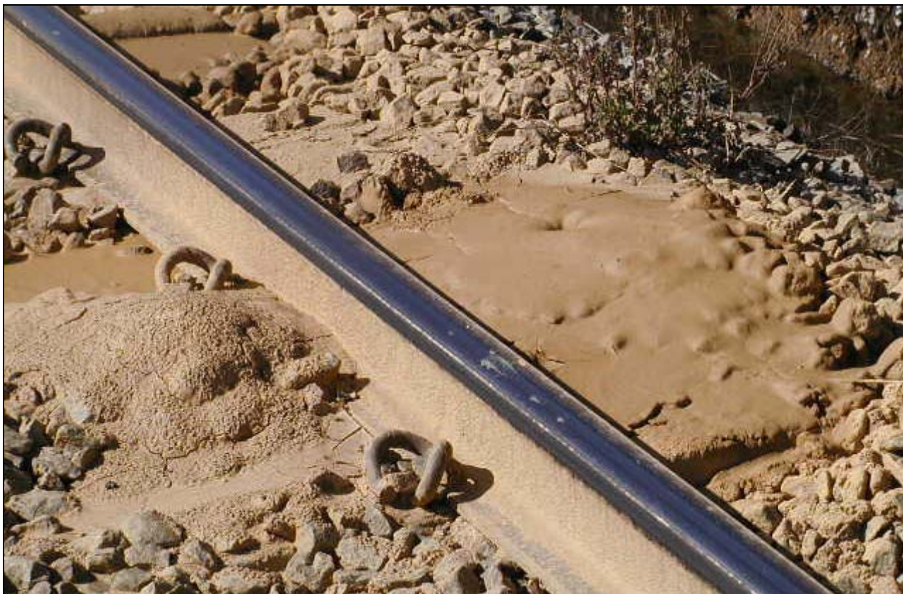
Figure 4-3: The presence of water and excessive track deformation pump mud to the surface
