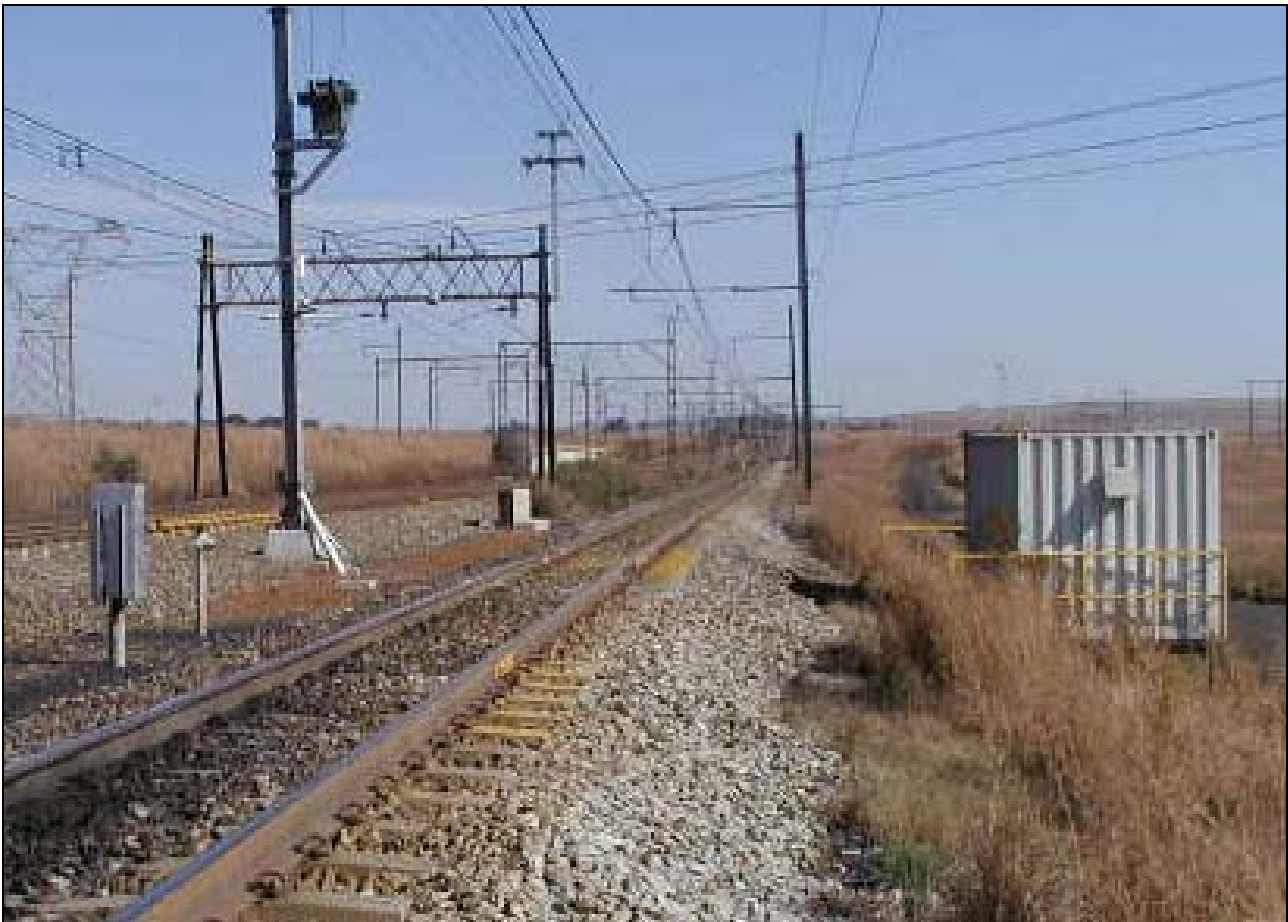
Figure 4-8: A complete unmanned weigh-in-motion weighbridge.
