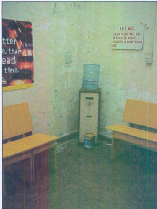
Figure 17: Capillary moisture (Source: Photo by author)
