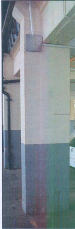
Figure 23: Brick column of D2 attached to concrete column of D1 (Source: Photo by author)
