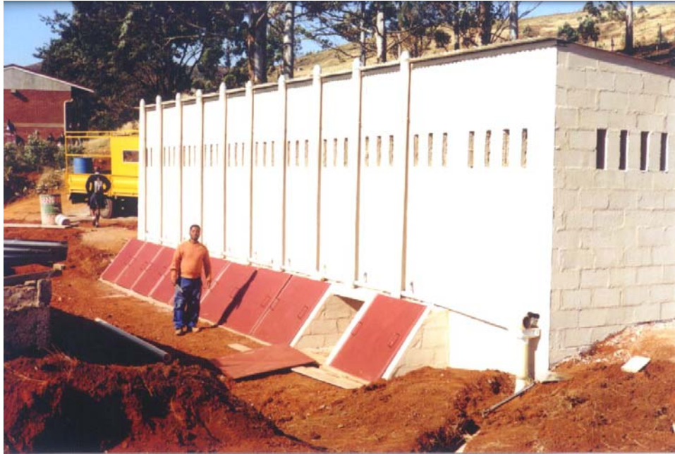
Figure 6.9: Well-fitting vault lids at a school toilet block (Photograph: CSIR)
