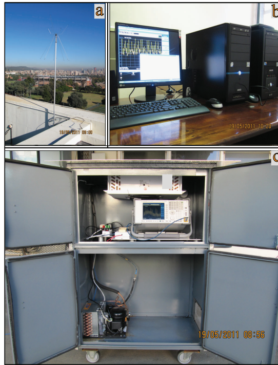
Figure 5.4: Photograph of the physical installation of the spectrum measurement system. Part a is the antenna, part b the storage and scheduler PCs and part c is the metal cabinet.
