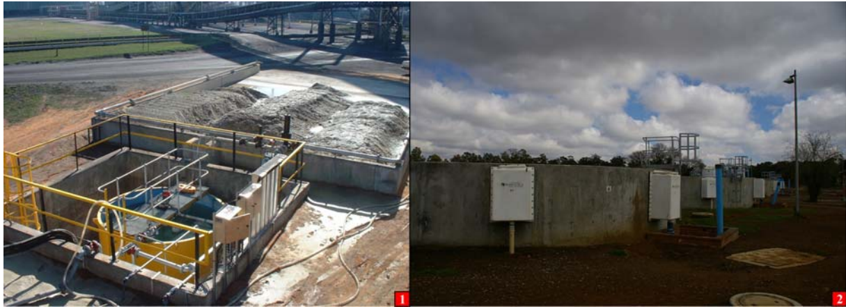
1 Limestone make-up facility at the Landau Colliery navigation plant (courtesy of A. van Niekerk, Golder Associates Africa).
