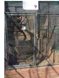
Figure 69. Steel frames and mesh protect the enclosures.
