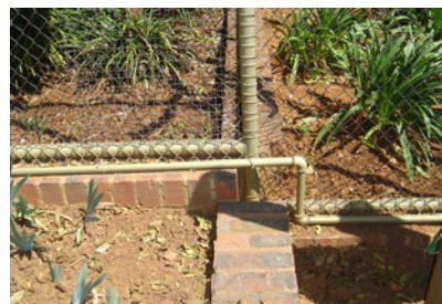
Figure 124. The enclosures' irrigation system. Water supply pipes run above to the middle of each enclosure.
