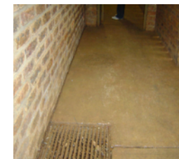
Figure 128. Drainage gratings in the Service Passage.
