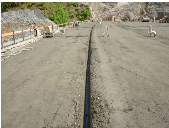
Plate 2.9: Instrumentation Cable Trench
