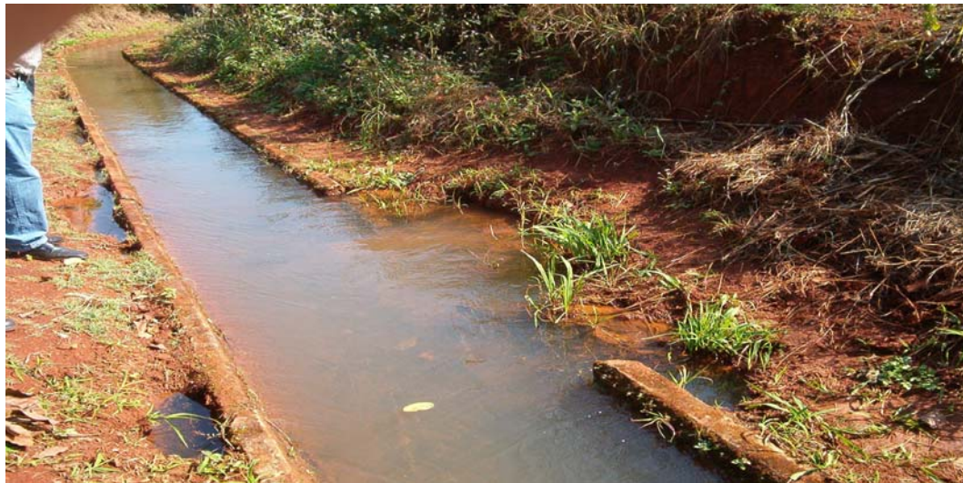
Photo 12.1: Poor maintenance of irrigation canals and excessive vegetative growth on the canal banks at Tshiombo Irrigation Scheme (irrigation blocks 3 and 4) causing inefficient water distribution
