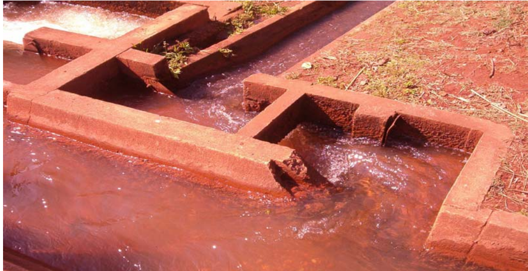
Photo 12. 2: Vandalism of irrigation delivery structures like a canal sluice gate at Tshiombo Irrigation Scheme prevent effective water distribution on the scheme (2003)
