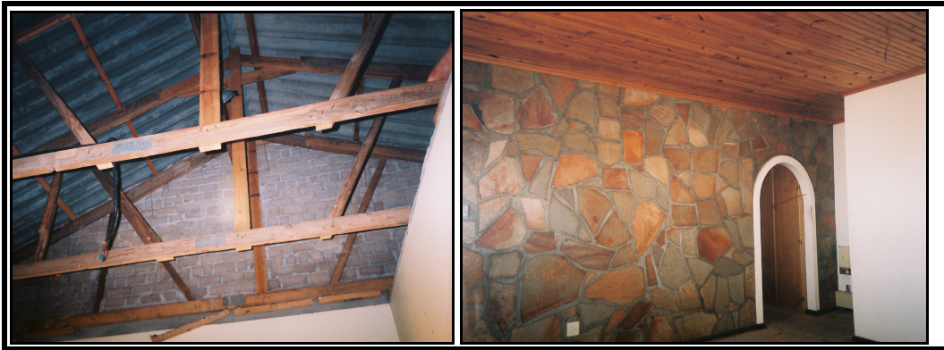
Figure 5.13: Condition of the farm house at Nanasan: Port Nolloth
