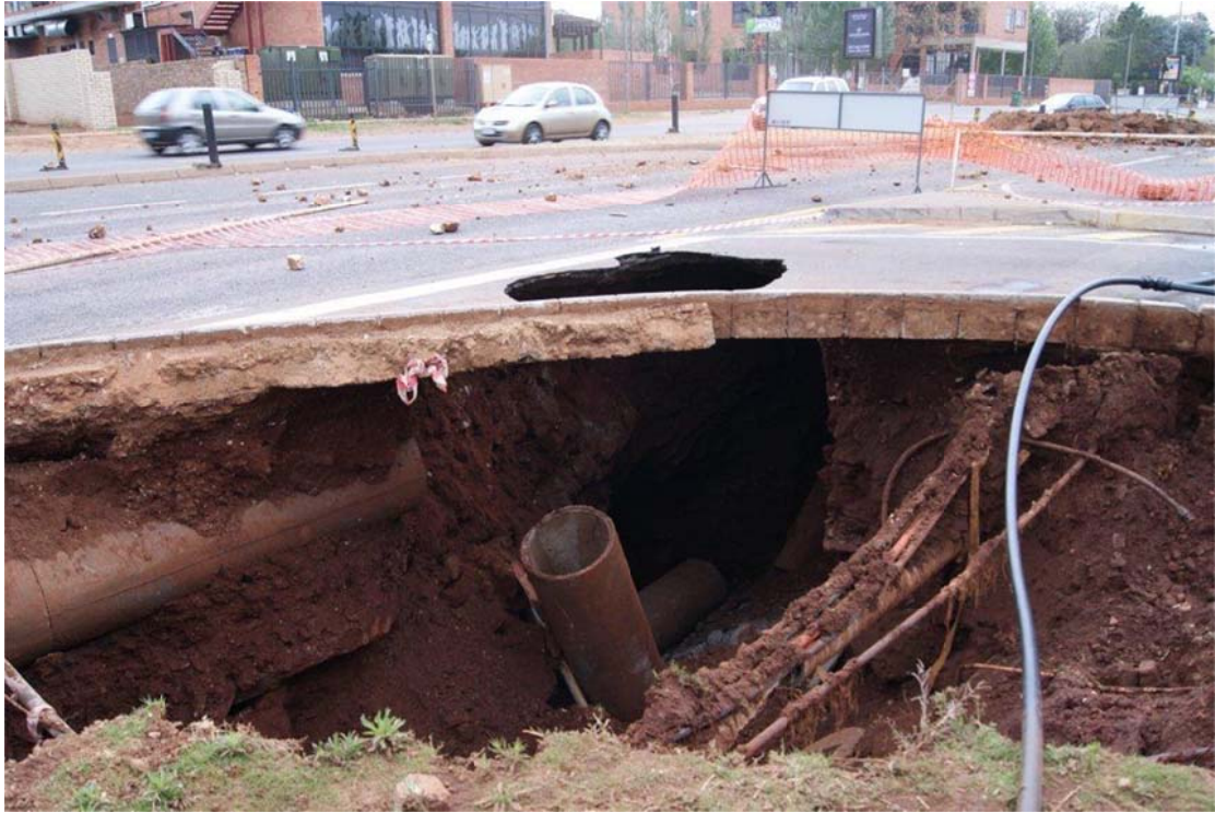
Plate 20. A Sinkhole that developed in Jean Avenue (S109)
