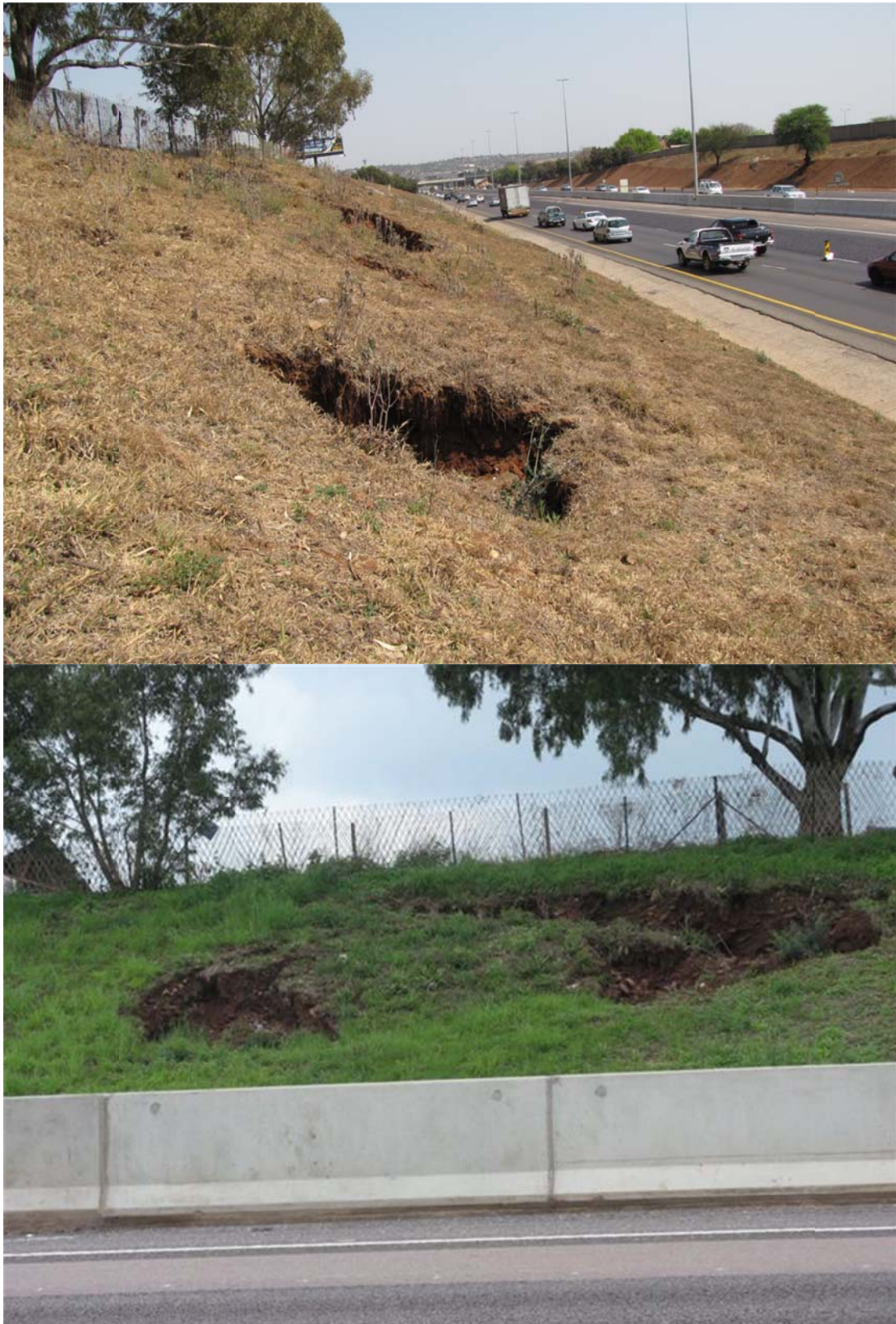
Plates 18 & 19 12 . Sinkholes that occurred on the embankment of the NI Highway (S104)
