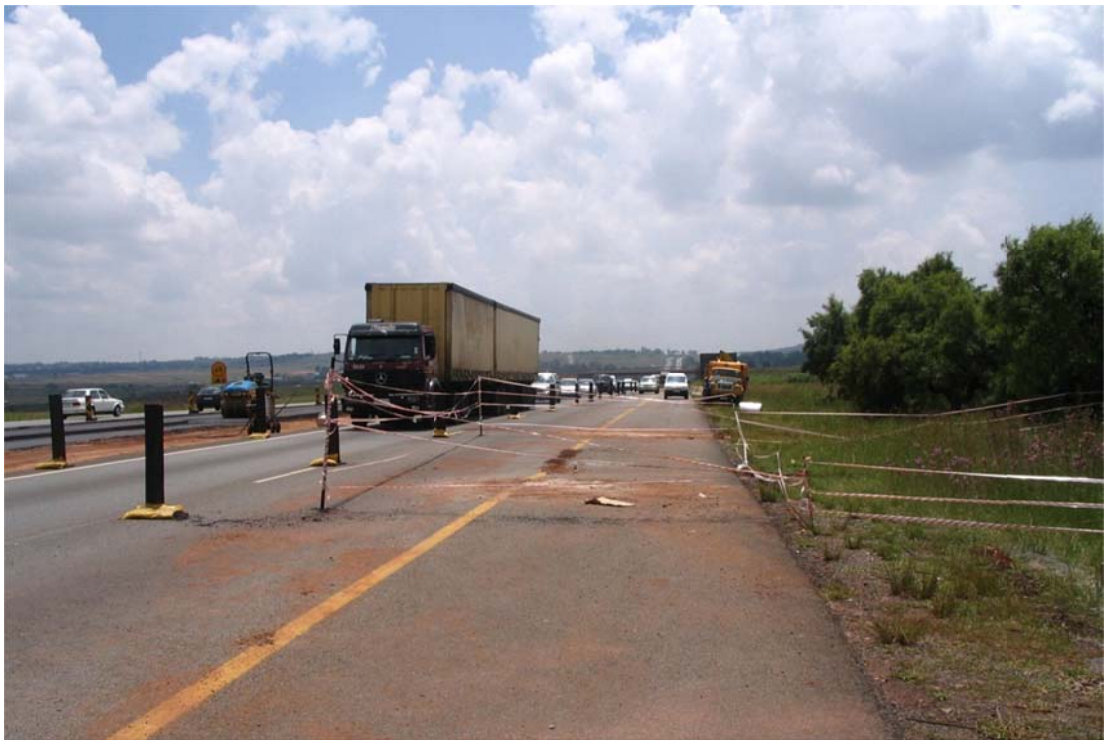
Plate 15. Sinkhole east of the N14 Highway (S101)
