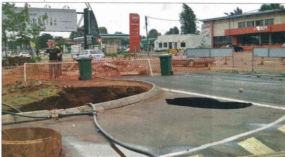
A sinkhole at the entrance to Jean Village. The earth caved in on Friday afternoon.
