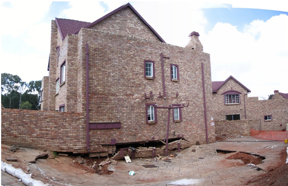
Plate 4. A 15 m diameter subsidence in a residential complex (S100)
