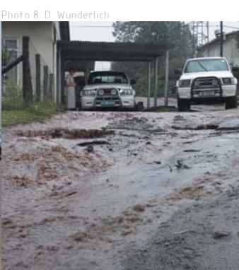
Storm water is a great problem, causing severe degrading of the roads.
