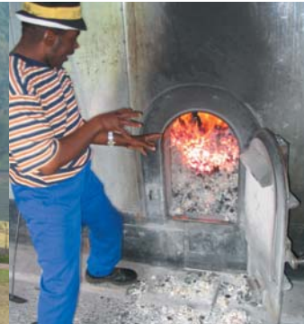
A coal boiler for water heating for part of the settlement.
