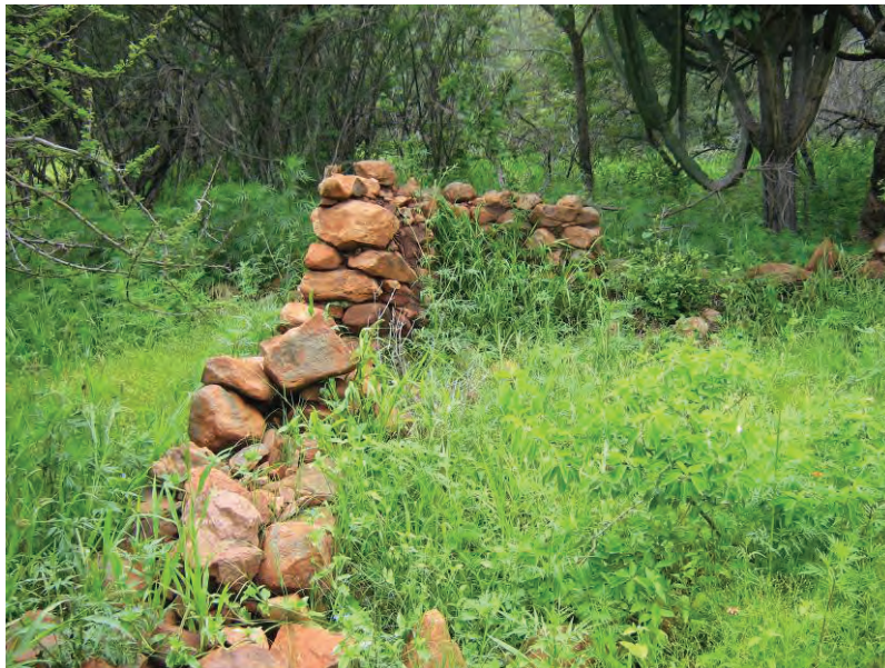
Figure 1 Example of a collapsed stone wall (source: photograph by the author).
