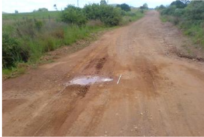
Figure 1: Condition of Rural roads in the Limpopo province.
