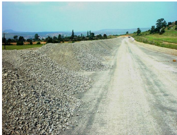
Photo 2: G1 material stockpiled on road.
