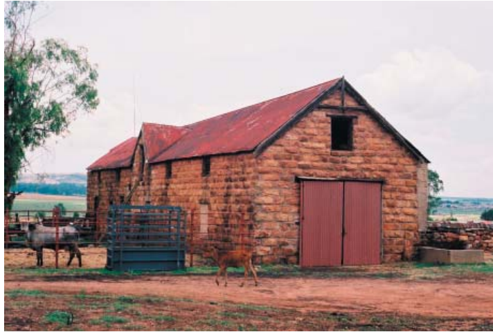
Figure 14 Sandstone ‘waenhuis’ and stables (for horses) on the farm De Rust west of the town of Heidelberg (Gauteng Province) (photograph: M. Naudé).
