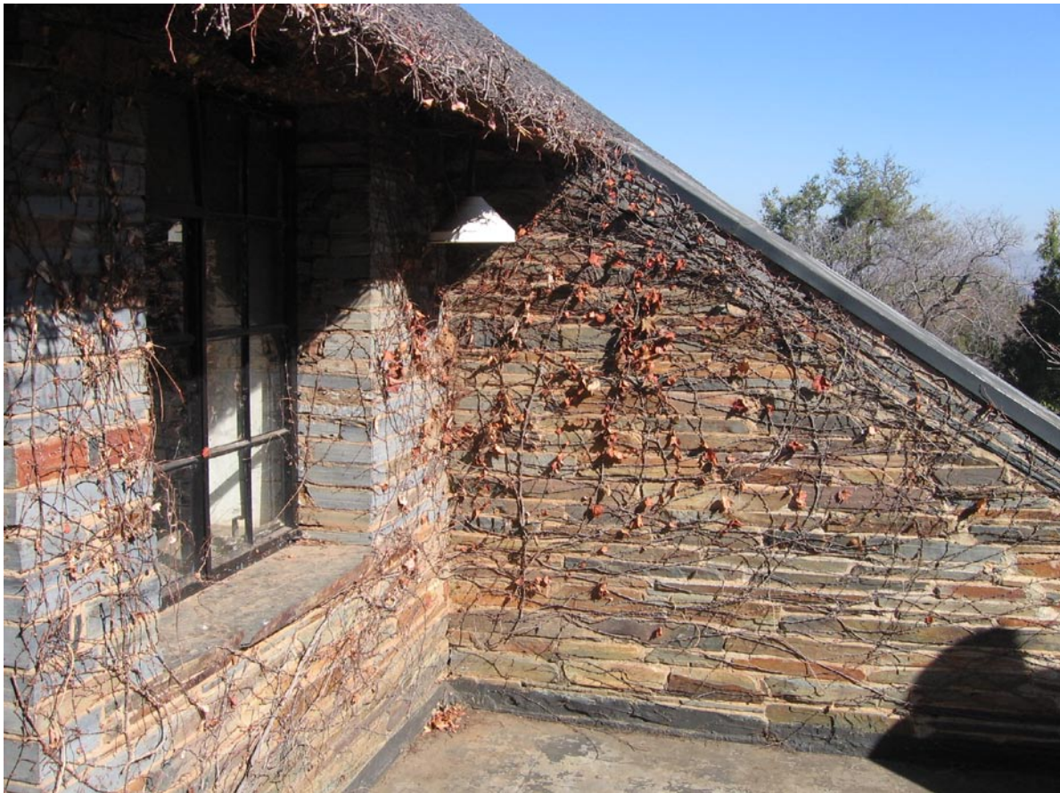
Figure 9 Detail of exterior and buttressing wall on the top storey of the Preller house (Pelindaba, Pretoria), constructed with slate. Finishing of diagonal buttress was done with long bars of slate (photograph: M. Naudé).
