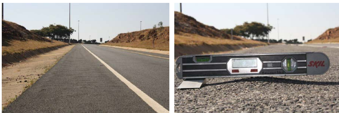
PHOTOS 1 and 2: Manifestation of small “bumps” on the surface in areas with low traffic volumes
