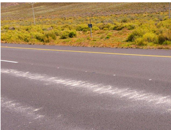
PHOTO 3 Cracking and pumping of fines through BRASO surfacing in the Western Cape
