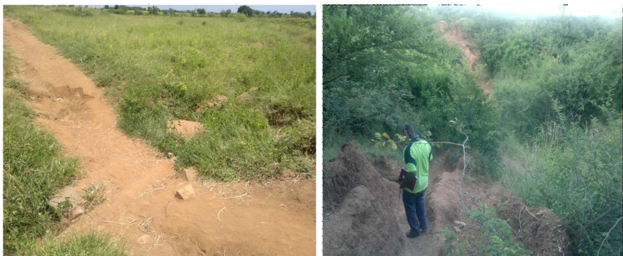
Figure 1: Sections of damaged local access roads and crossing points in Masia
