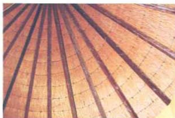
Fungal growth on the inside of a thatched roof in Durban
