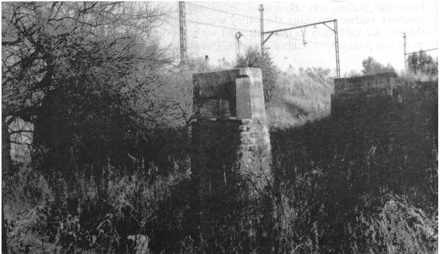
Central pillar and western abutment of the old Moreletta Spruit railway bridge on the eastern side of Pretoria
